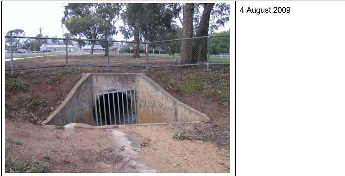
Figure 4-3 Entrance to the piped section of the Maddingley Park Drain (near the corner of Griffith St and Parwan Rd)
