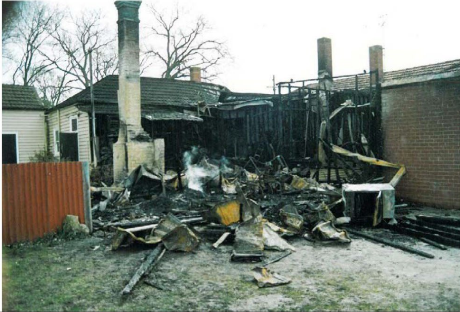
Figure 3: Fire-damaged Bridge Hotel from the rear, 1992.
