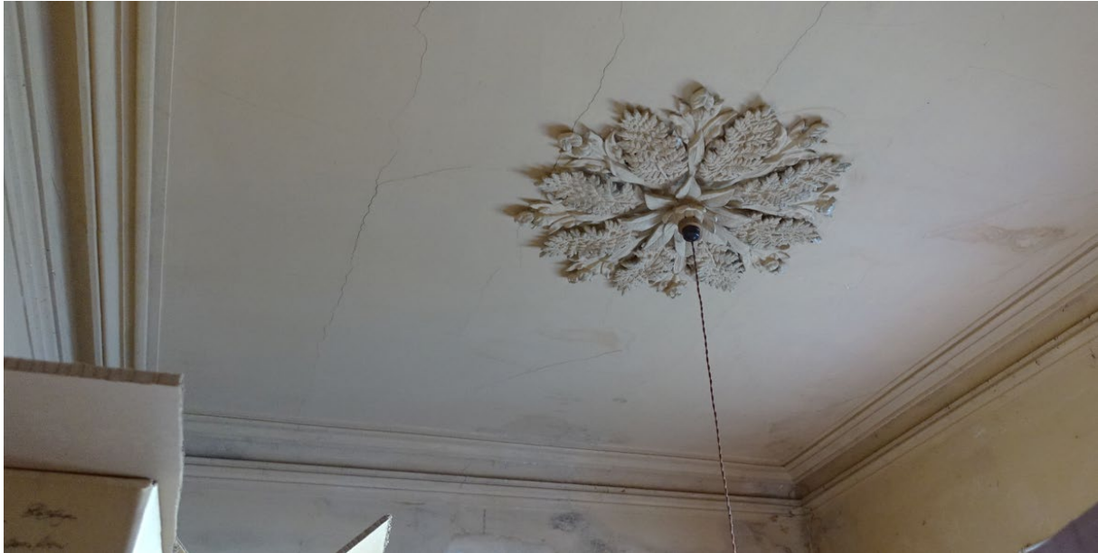
Photo 9: Ceiling, cornice and ceiling centre in the north-east ground-floor room, 2025.
