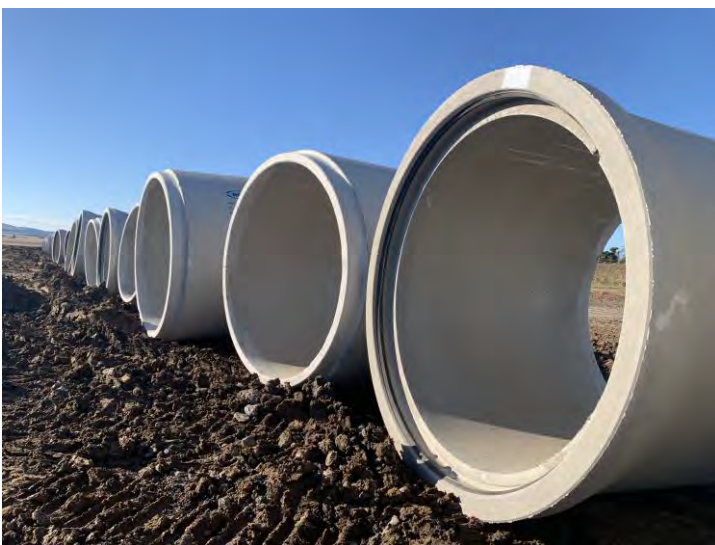
Figure 54. Rubber Ring Jointed pipes on other sodic soil sites
