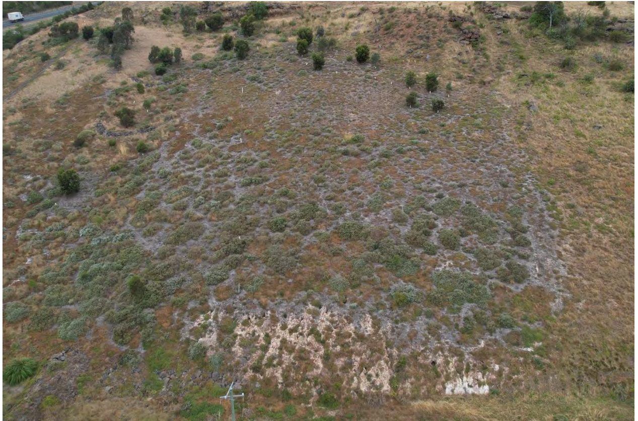
Image 26 – Aerial view of failing fill (grey and white material), located north west of subject site in DOTP road reserve.
