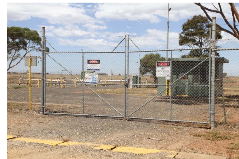
Photograph 9: Brooklyn-Ballan gas pipeline at Rowsley Park Road
